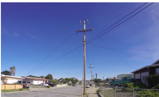
1b. Coaxial and telephone wiring of neighborhood
